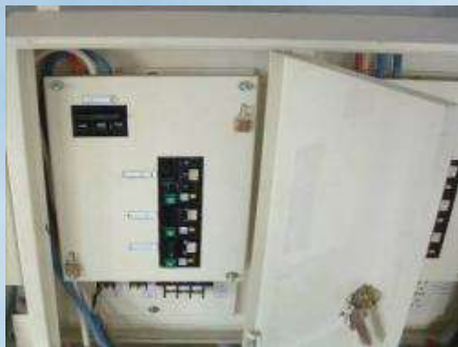
Use electricity leakage breakers
